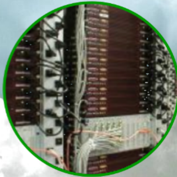
Purpose built hardware
