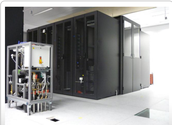
Enclosure and "Cooltrans"
