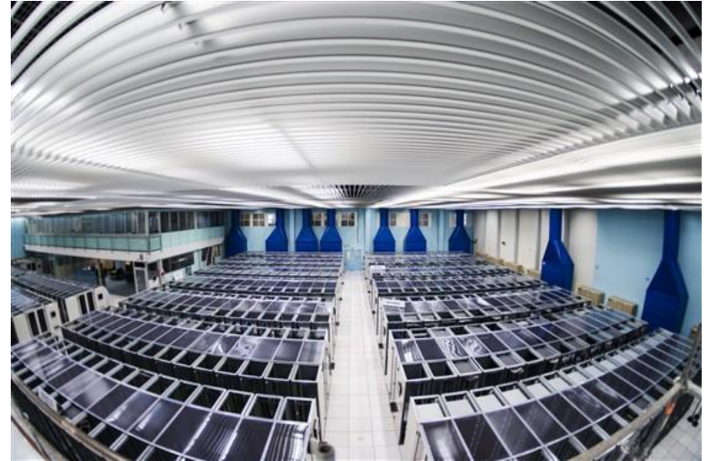
CERN's Computer Center (1st floor)
