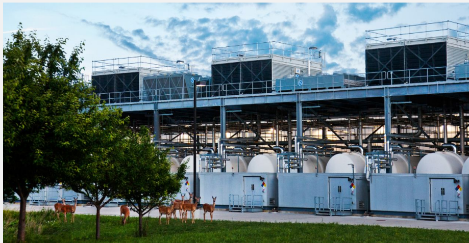
Council Bluffs, Iowa. Google Data Center. Photo: Google/Connie Zhou.
