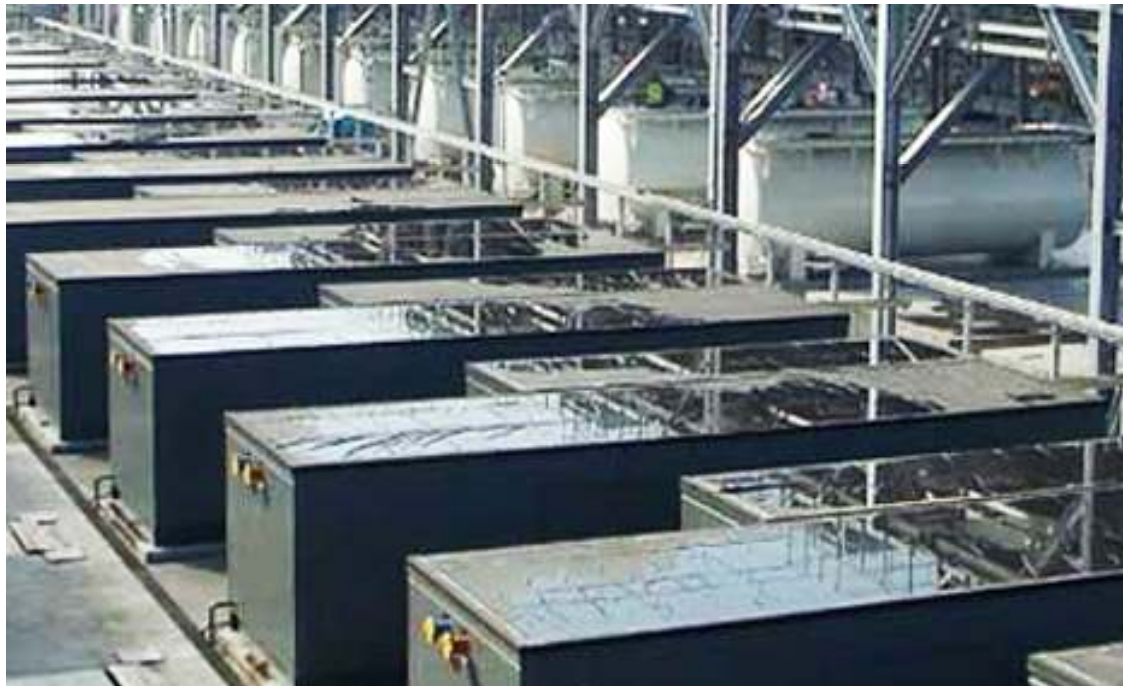
Google Data Center in Belgium
